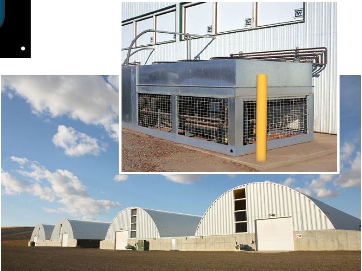
Storage Climate Controls
